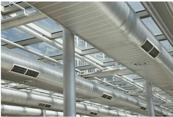
Figure 9. Air Conditioning Ducts in a Large Building
